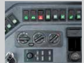
Instrument Switch Panel
