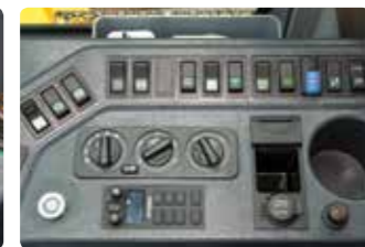
Centralized Instrument switch Panel
