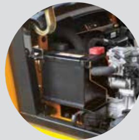
Rotational Battery Installation
